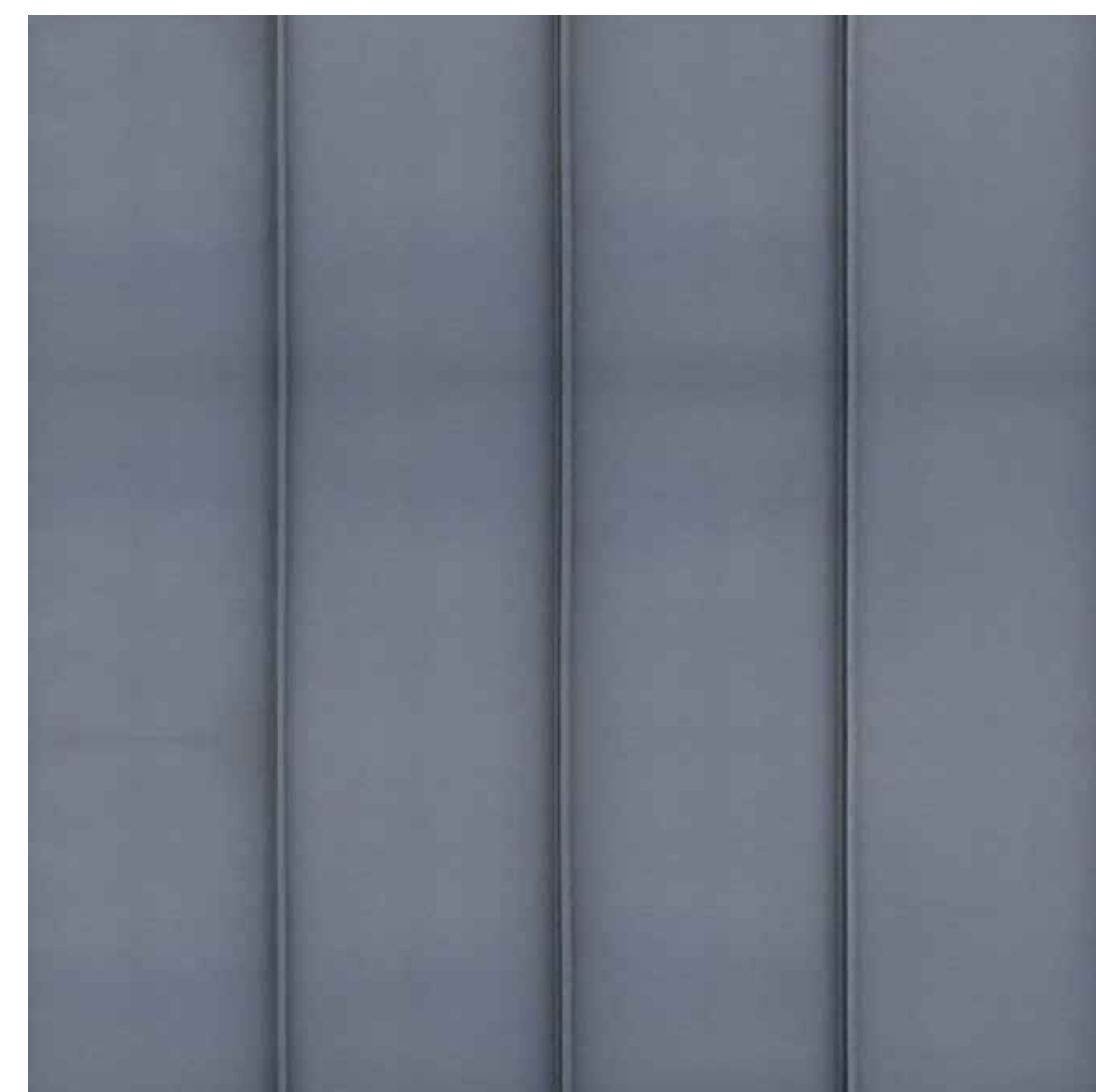
6) Zinc At chimneys & parapet caps
