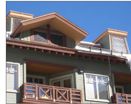
Group and screen mechanical units from view.
